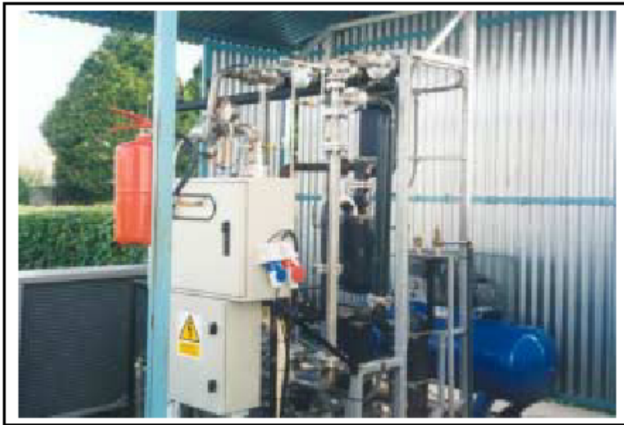
Figure 14: University of Nottingham ejector cooling system capable of heating, cooling, and electrical power generation.
